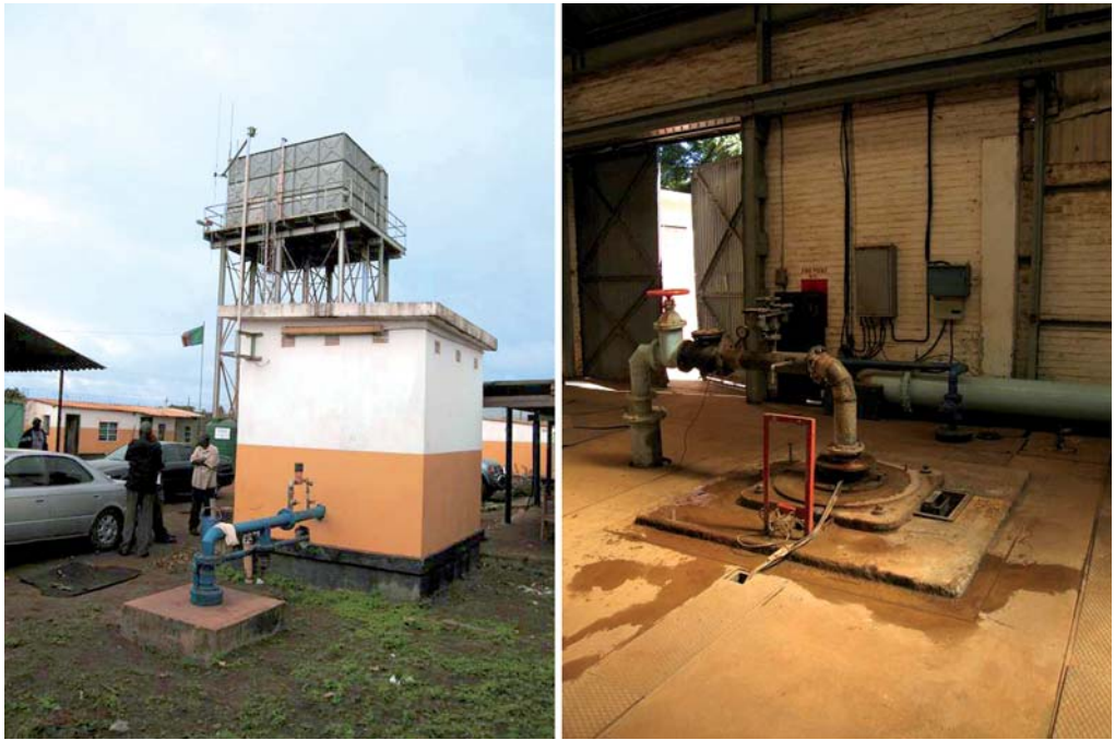
Figure 19: Municipal water supply wells in Lusaka.
