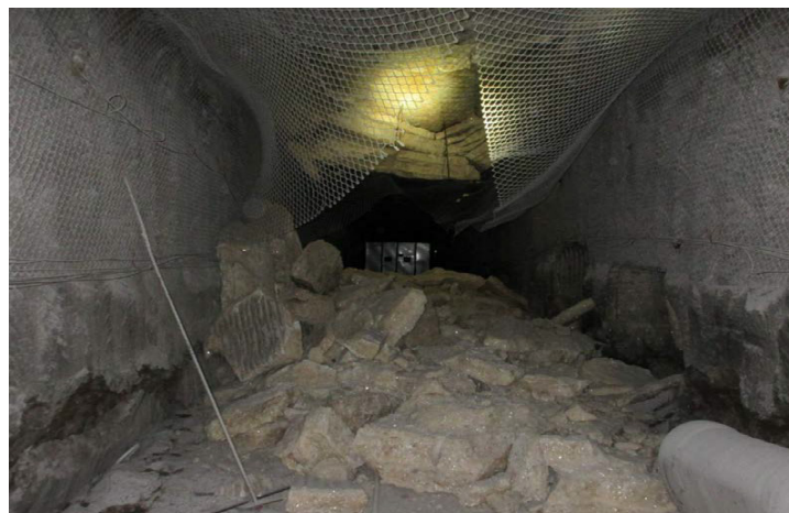
Figure 4.2: Roof fall in Panel 3 access drift at WIPP.
