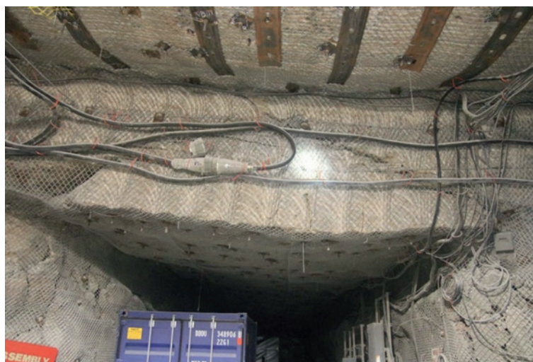
Figure 2.3: For the second demonstration model, a drift with slab separation above the sealing was suggested. The photo shows a crack above a drift at WIPP.
